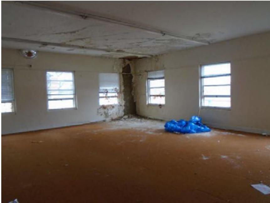
Photograph 11: Overall view of second floor with moisture damage along exterior wall.
