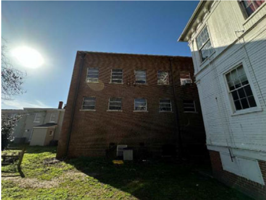
Photograph 15: Overall view of left (North) elevation. No control joints observed. Cut in masonry control joints.
