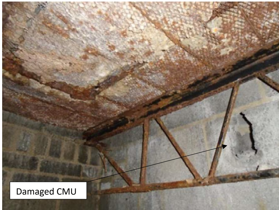
Photograph 5: A close-up of open web joist with significant corrosion. CMU is also damaged. Square off area of damage and mortar in a new face shell.
