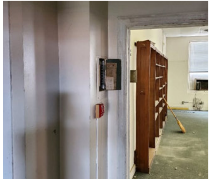
Elec Photo #3: Load Center Recessed in Elevator Lobby Wall
