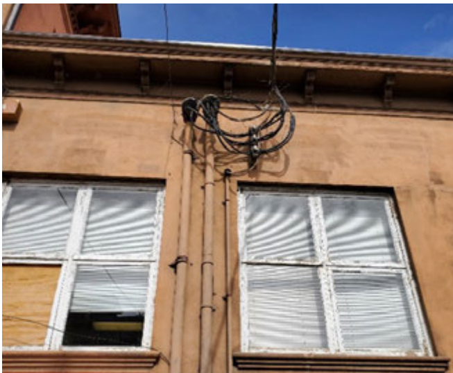
Elec Photo #1: Overhead Service Drop & Exposed CTs
