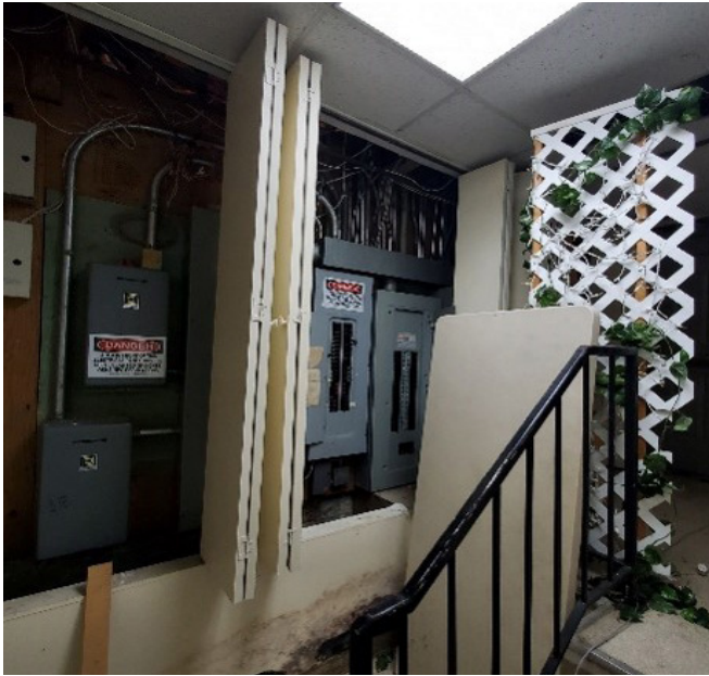
Elec Photo #2: Existing Main Electrical Closet
