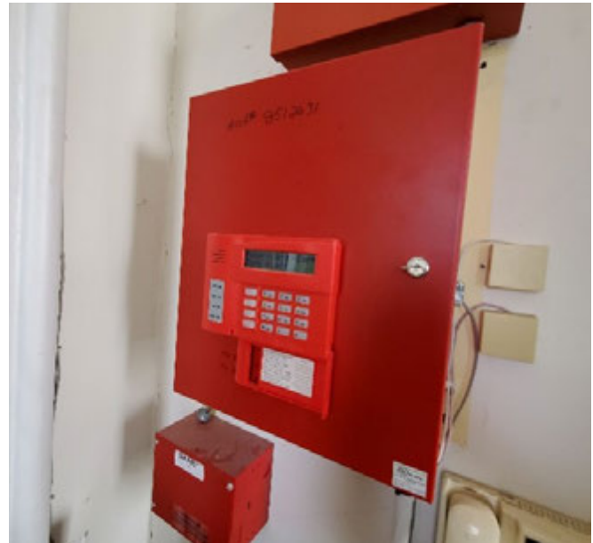
Elec Photo #8: Existing Combo Fire/Security Panel
