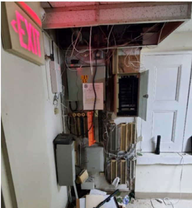
Elec Photo #9: Existing Telecom Backboard & Headend Equipment
