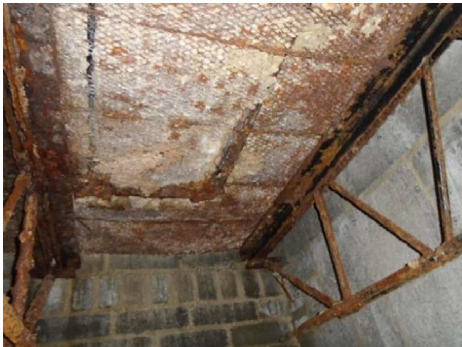
Photograph 6: A close-up of open web joists with significant corrosion. Install W12x14 beams adjacent to affected joist. We recommend shoring the floor prior to the renovation work to protect the public.
