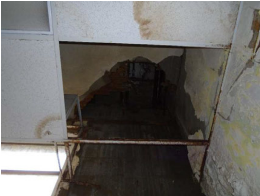
Photograph 10: A close-up of second floor open web joist with corrosion.
