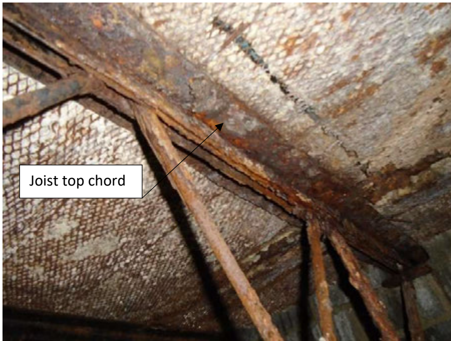
Photograph 8: A close-up of open web joist top chord with significant corrosion. Top chord is 75% deteriorated. This is a safety hazard and requires reinforcement. Install W12x14 beams adjacent to affected joist. We recommend shoring the floor prior to the renovation work to protect the public.
