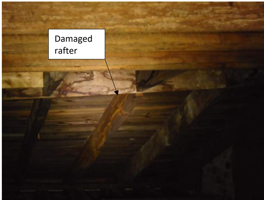
Photograph 13: A close-up of damaged roof rafter. Sister by adding 2x8 rafter along the damaged rafter fastened to the existing damaged rafter.
