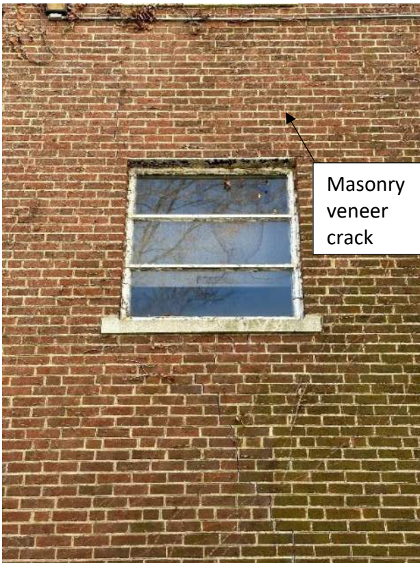
Photograph 17: A close-up of masonry veneer cracks. Cracks are the result of non-existent masonry control joints. Install masonry control joints.
