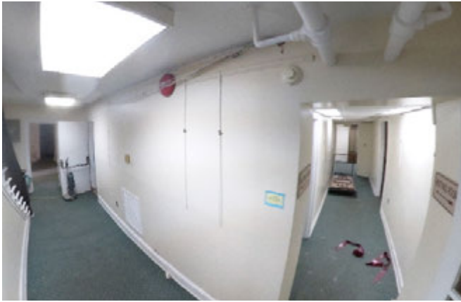
Elec Photo #4: Exposed cabling in Corridor
