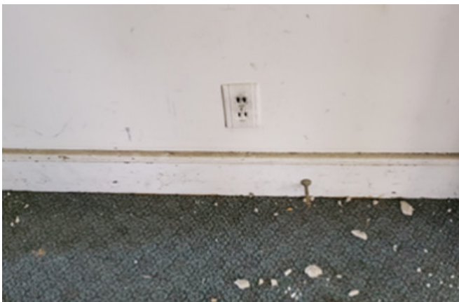
Elec Photo #5: Receptacle, No Ground
