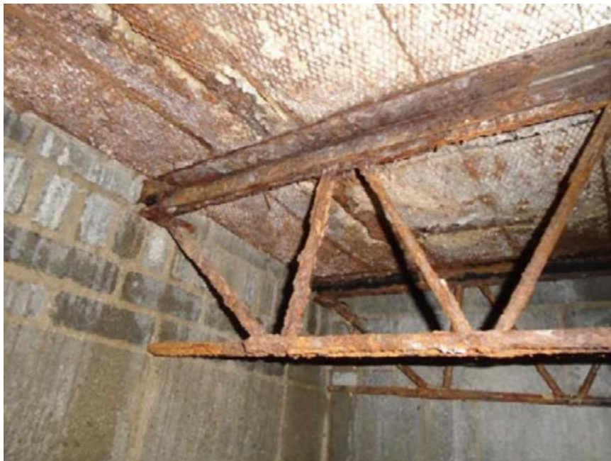
Photograph 4: A close-up of open web joists with significant corrosion. Install W12x14 beams to adjacent affected joist. We recommend shoring the floor prior to the renovation work to protect the public.
