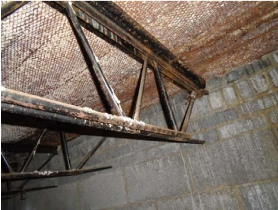
Photograph 7: A close-up of open web joists with moderate corrosion.
