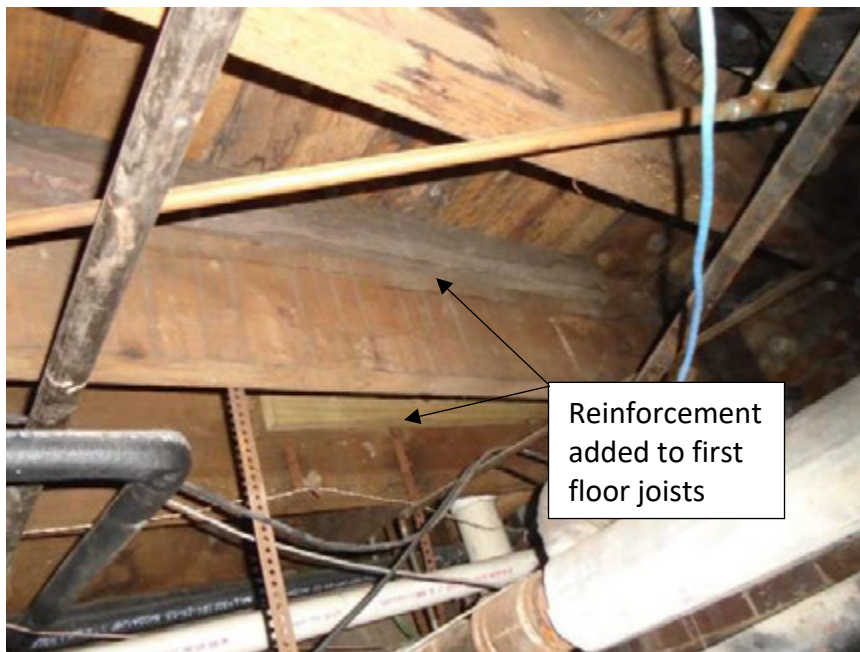
Photograph 14: A close-up of reinforced floor joists where joists is split. Sister by adding 2x12 floor joist along the damaged joist fastened to existing damaged joist.
