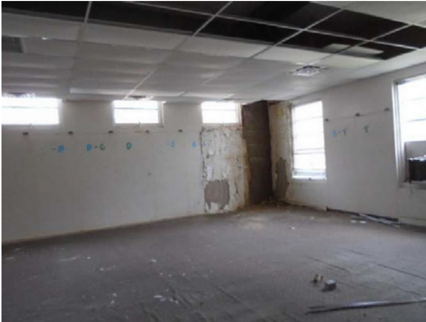
Photograph 9: Overall view of first floor with moisture damage along exterior walls.
